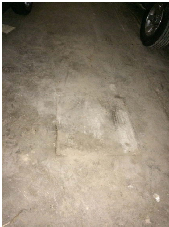
Photo #4: Concrete patch in concrete inside building
