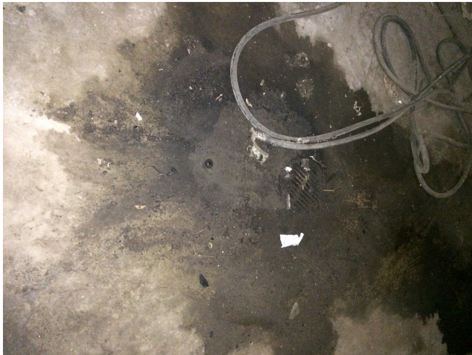
Photo #2: Staining of concrete surrounding drain in northwestern portion of building
