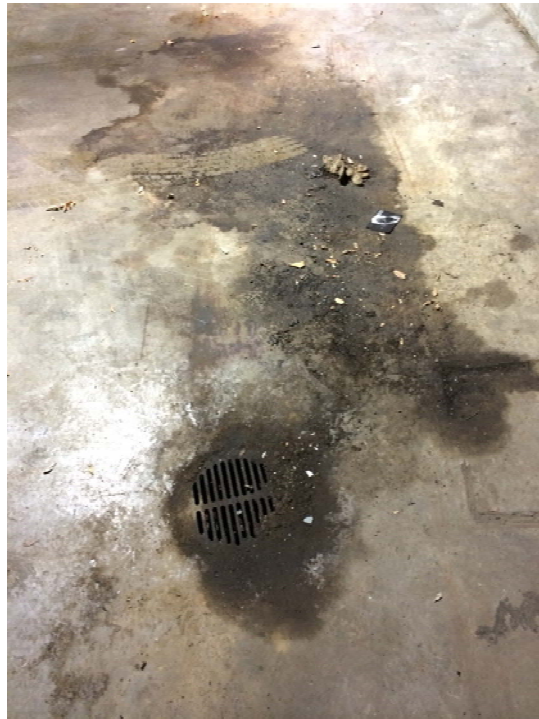
Photo #3: Staining of concrete surrounding drain in southeastern portion of building
